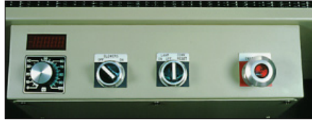
System control panel.
